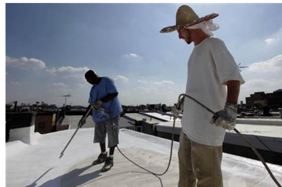
James Peterson, left, and Rory Stout of Bio Neighbors apply white paint to a roof in Philadelphia.
