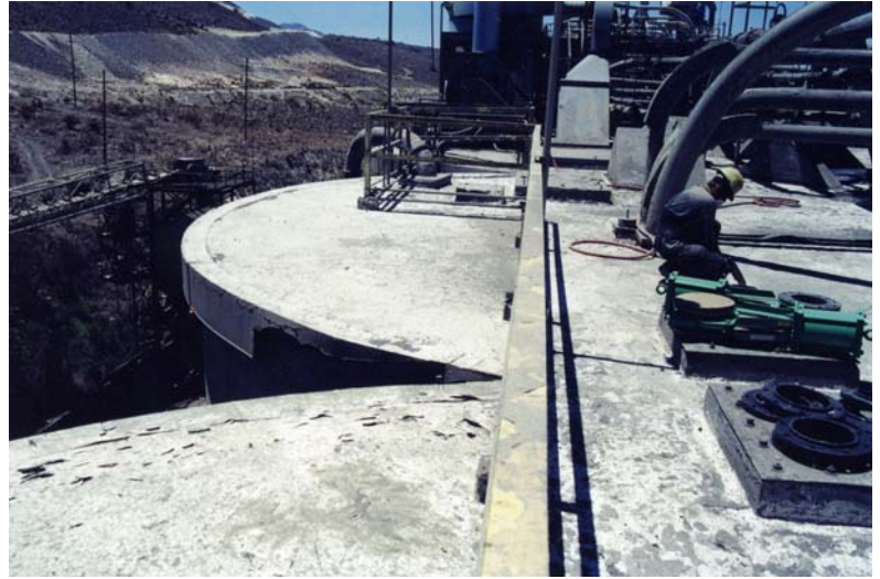
The roof deck stripped of cement. It is now ready for priming
