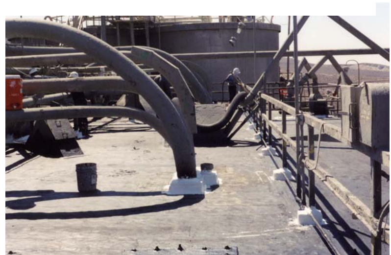
After the roof deck was primed all pitch pockets, boxes, flashings and equipment was sealed with Acu-Caulk and Acu-Fabric polyester by Energy Seal Coatings, Inc.
