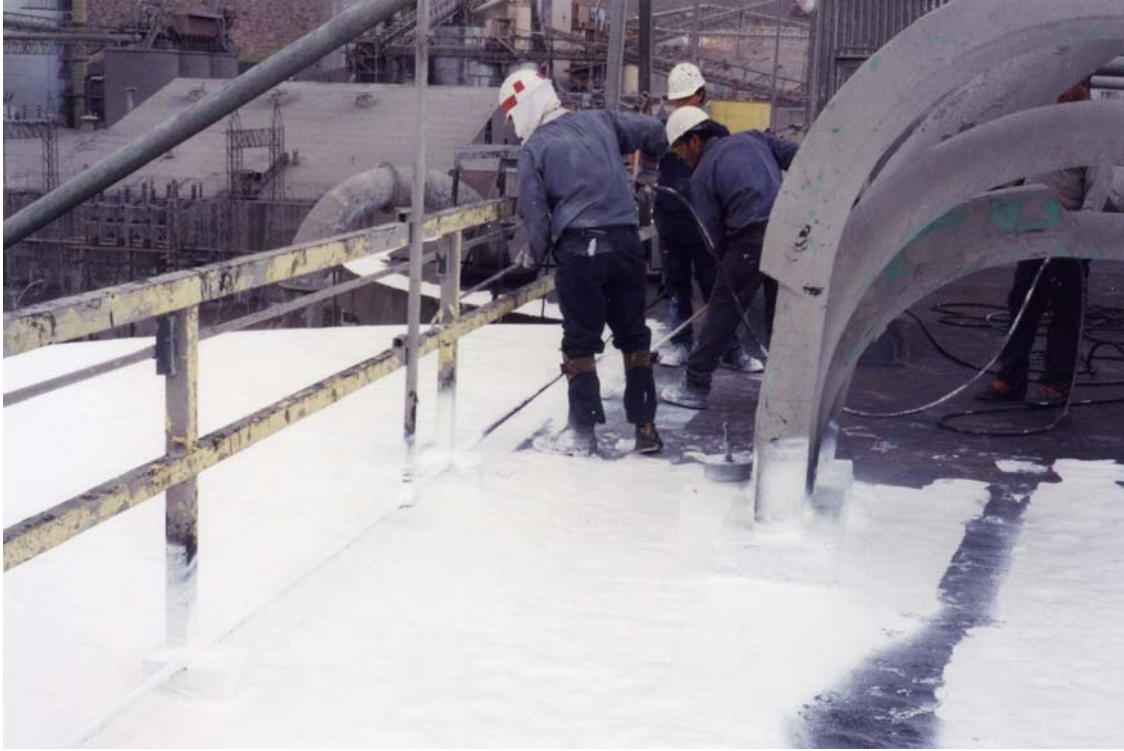
Spraying the first layer of Energy Seal's Acu-Shield onto the roof deck
