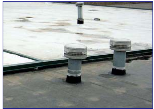
Figure 3 – Photo of roof on December 15, 2003. The PVC membrane is on the top, in white; the EPDM membrane is in the foreground.
