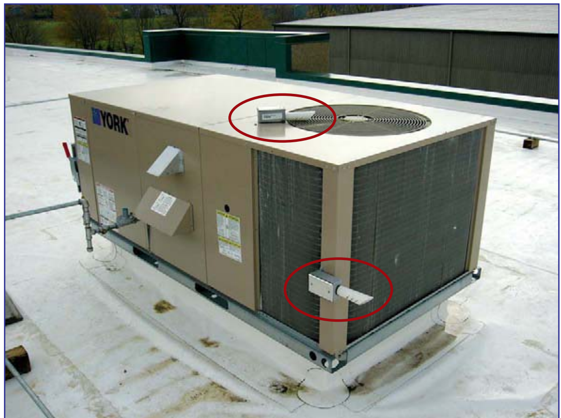
Figure 9 – York HVAC unit with sensors (circled).
