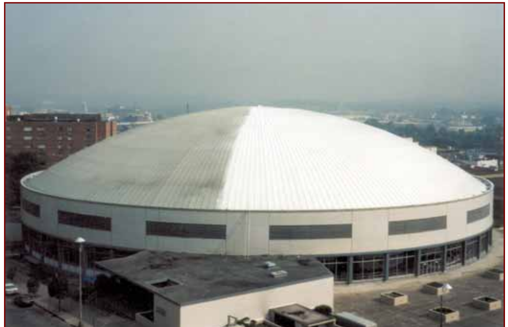
This metal roof at Eastern Tennessee State University is partially covered with a white coating. The coated half of the dome contrasts sharply with the uncoated half mid-way through the application process.
