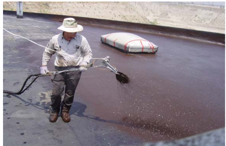
Fiberglass roving is chopped through a special gun at the same time the emulsion is applied. This creates a thick waterproof barrier that water cannot penetrate.
