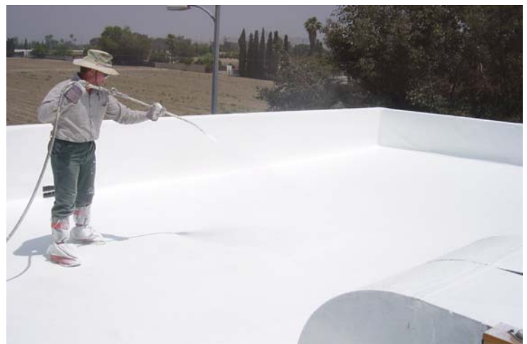
2 layers of Acu-Shield white coating are sprayed onto the roof. This will reduce temperatures and save money.
