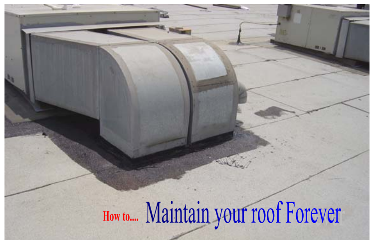
All penetrations are primed to create a solid long lasting bond to the new maintenance roof.
