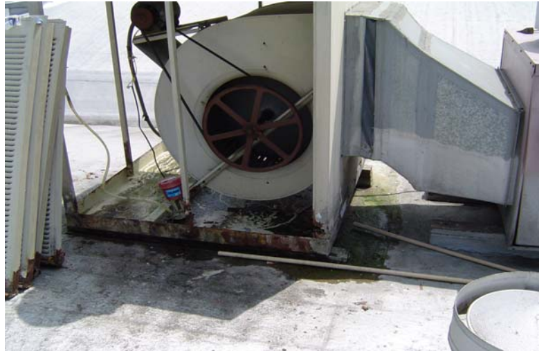
This old swamp cooler was removed. A new one was to be installed after the roof was coated.
