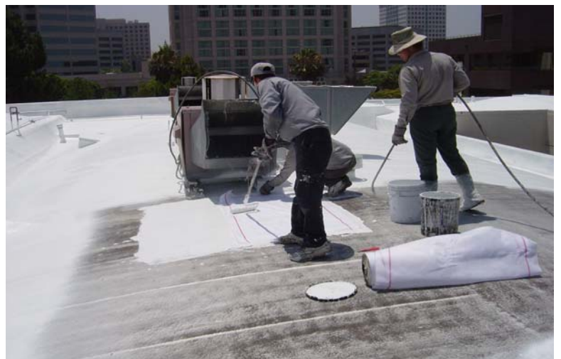
Applying the final layer of Energy Seal elastomeric over the repaired area.
