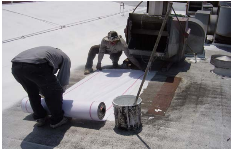
Polyester and an elastomeric caulking was installed where the old swamp cooler sat.
