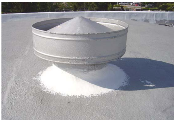
All pipes and vents were flashed with Energy Seal's Acu Caulk: Brush Grade.
