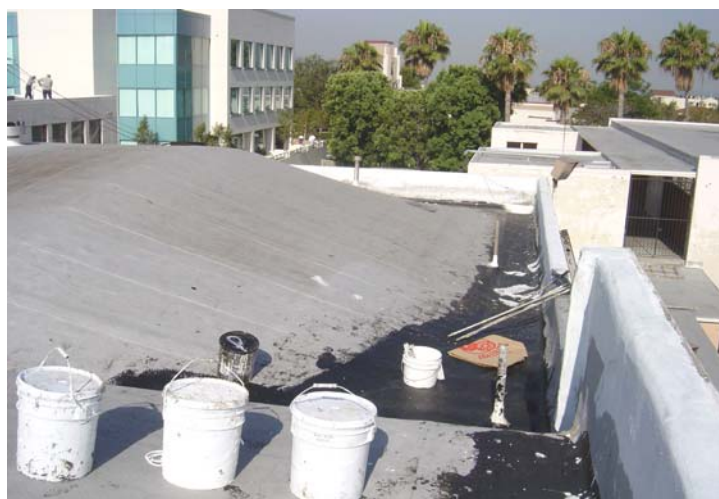
The valley areas were reinforced with an extra layer of polyester and emulsion.
