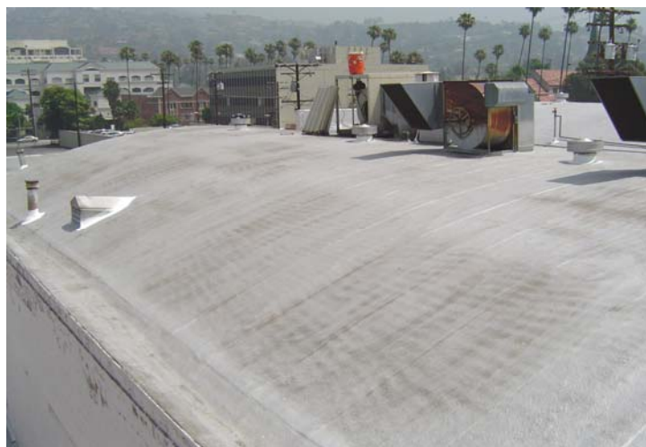
After 11 years the roof does not leak and is still in waterproof condition despite the fading aluminum
