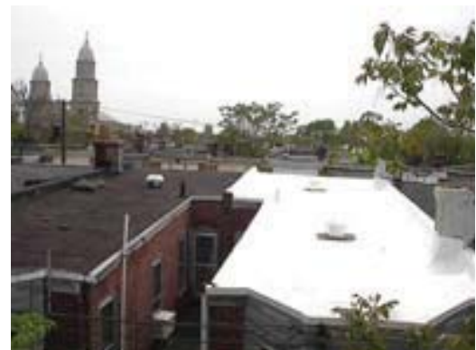
This residence contains white roof coatings which is representative of the refurbished homes participating in the Philadelphia “Coolest Block” contest. Photo courtesy of Dow Chemical Company.
